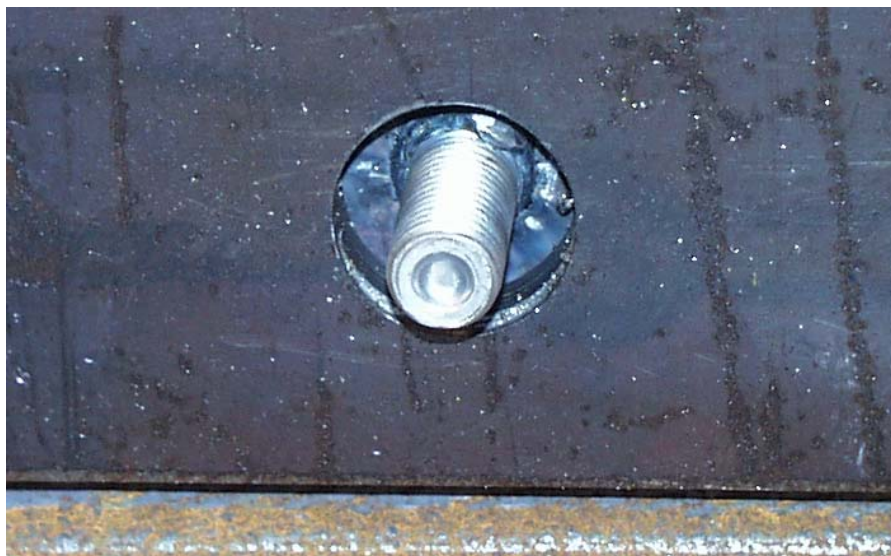
Figure 6.75 Gap around threaded stud
